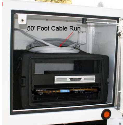
A 6RU rackmount case is locked behind a stainless steel weather-proofed trailer cabinet door. The rackmount case itself can be moved up to 50 feet from the trailer, and placed inside of a structure or tent if desired.
